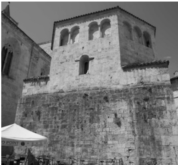
Baptistry of San Giovanni, Ascoli Piceno, Italy, ca. twelfth century, view showing masonry breaks on east exterior wall (photo: Joseph Williams).
